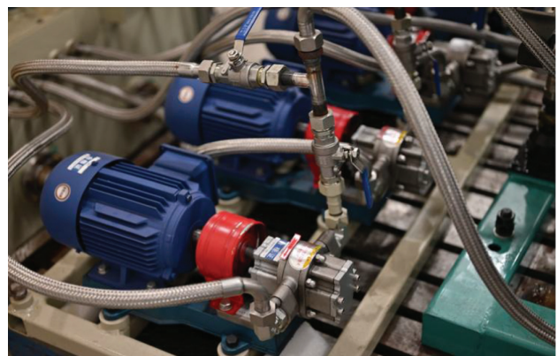
Fig. 5. The oil-feed pumps.
