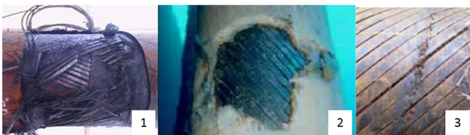
Fig. 2. Riser damage: (a) armor wire breakage, (b) external sheath damage, and (3) armor corrosion.
